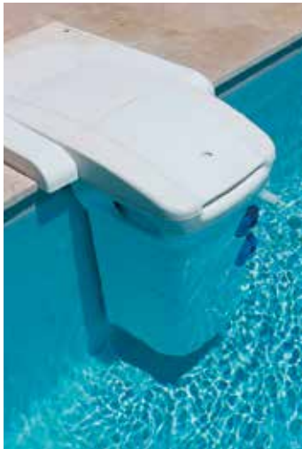
Straddle filtration unit (GR.I 181)
